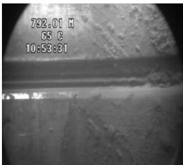
Here the ViewMax examines a collar which has failed a pressure test
