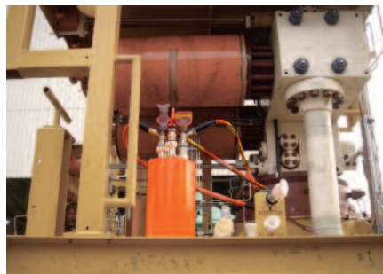
CaTS subsea receiver on subsea tree
