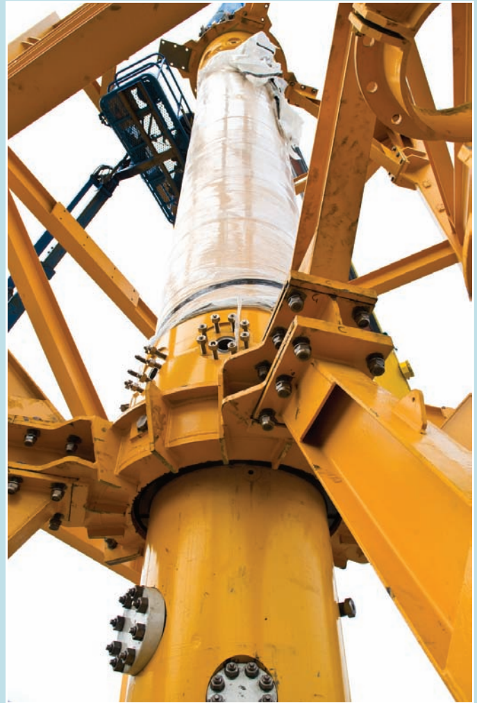
TSP pressure housing installed in frame
